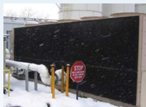
The same York chiller with durable, cleanable PreVent equipment protection filters.
