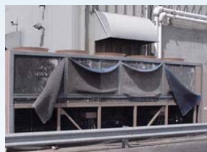
A York chiller with ineffective, disposable filters.
