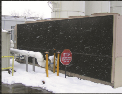
Automated Packaging Plant 200 Ton Chiller
