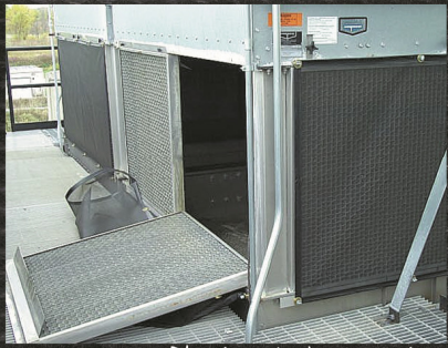
Physics Laboratories HVACR Equipment
