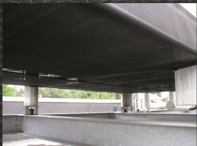
Jackson National Life Facility Dry Cooler Rooftop Unit
