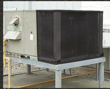
Physics Laboratories HVACR Equipment
